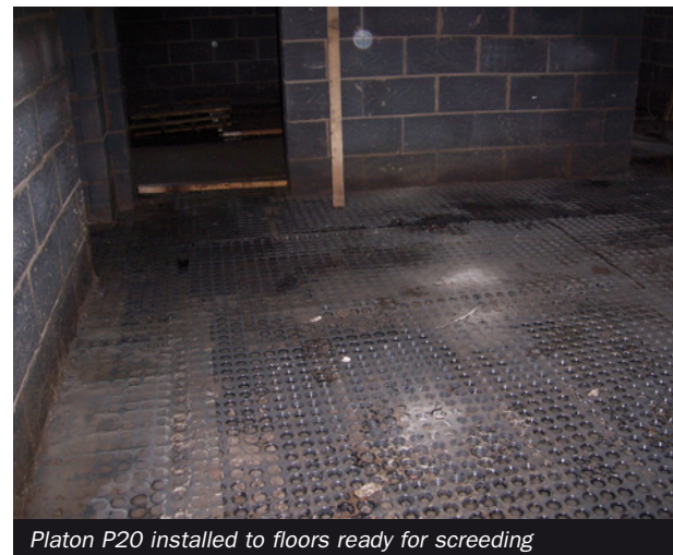
Platon Multi was installed after the application of TT Vapour Membrane as an anti lime coating
