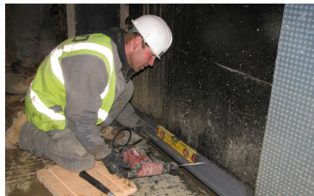
Checking the fall of the Triton Aquachannel, installed around the perimeter walls, to divert any water from behind the membrane system to the discharge points
