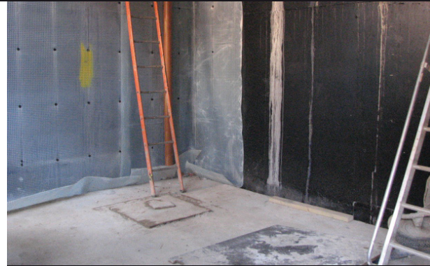
Cavity drain membranes were installed on the concrete walls after the application of two coats of TT Vapour Membrane
