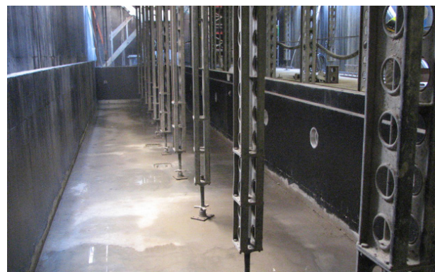
The concrete walls and floor of the swimming pool were waterproofed with TT Vapour Membrane before tiling
